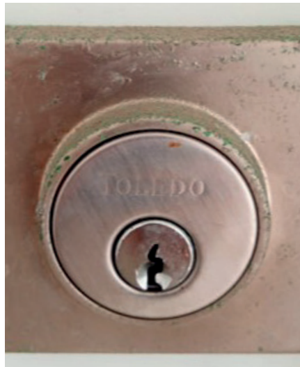
Abb. 13: DOOR LOCK, affected by rust, 2020
